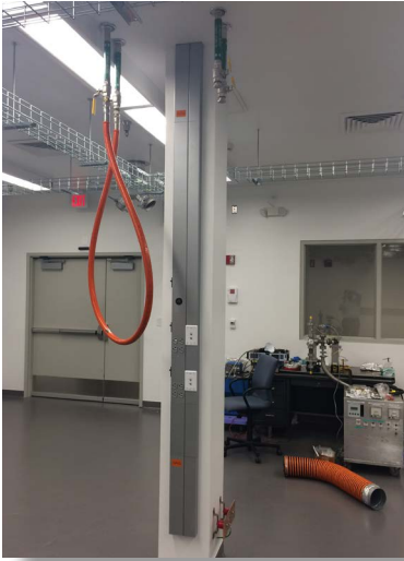
60 amp Plug-In Raceway Power & Data system installed vertically for additional outlets
